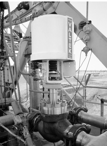
This cryogenic Mark One is used for aerospace testing as an O 2 vent.
