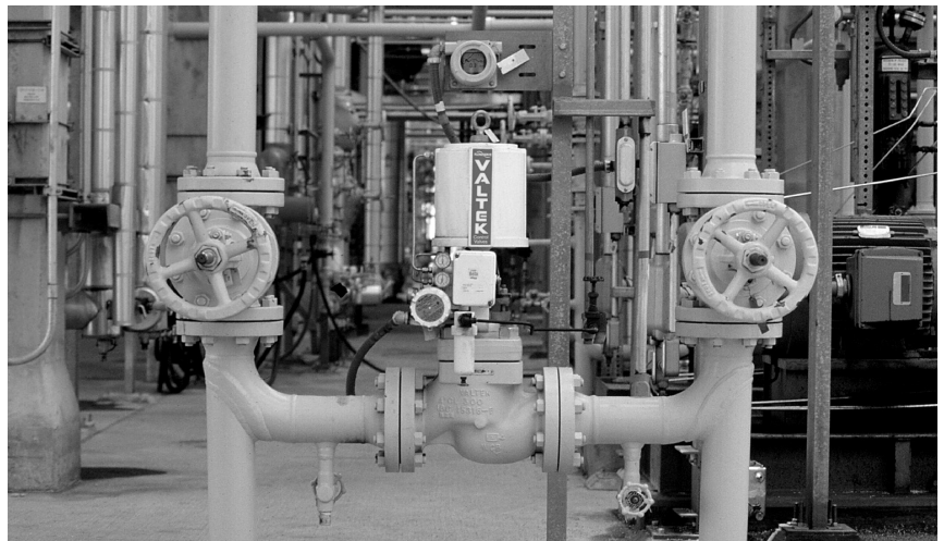
This 8-in, back-pressure control valve operates in a liquid hydrocarbon plant with a 580 psi/40 bar upstream pressure.
